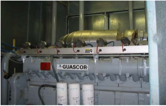
290-kW engine retrofitted to run on biogas, from Belgium-based Continental Energy Systems
